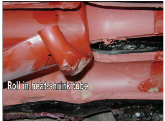
Heat-shrink joint improperly installed.
