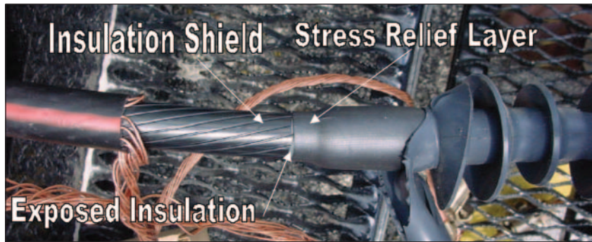
Stress relief portion of polymeric termination not overlapping onto cable insulation shield.
